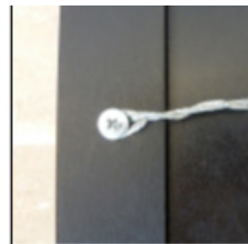
Unacceptable hanging hardware:
